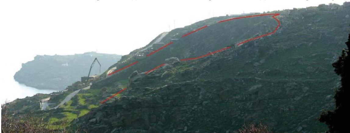
Photo 11. Rock falls and rock slide in the Aprovatou village area.
