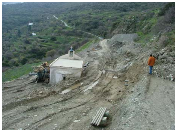
Photo 8. Destruction of a road and small church located downslope, near the village of Kochilou.
