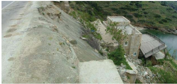
Photo 9. Severe damages of a villa built downslope from the road connecting the villages of Batsi and Gavrion. The cast in situ piles for the protection of the road pavement are also distinguished.
