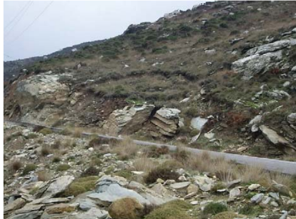
Photo 7. Rotational slide in weathering mantle of schist formations, with marble intercalations, affecting a road axis.
