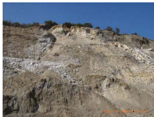
Fig. 11. Landslide at ch.9+700 along the road.
