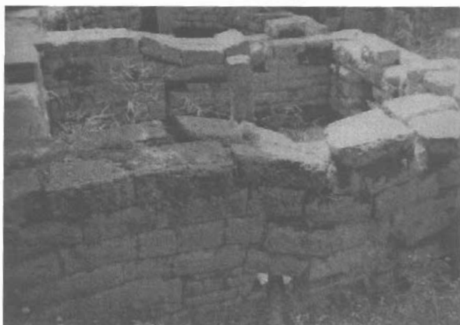
Fig. 7. The 4 th to 2 nd century BC Tower Gate (inner part). The most typical example of earthquake destroyed walls and foundation probably due directly to seismic fault activation, that is cracks (arrows) and tilted side (right) of the foundation.
