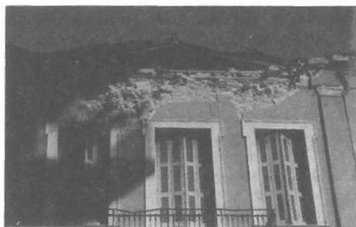
Fig. 9: Cracks on brittle structures in the city of Patras.
