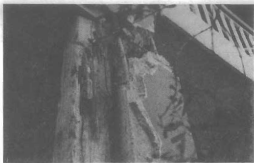
Fig. 8: Damage on reinforced concrete construction.
